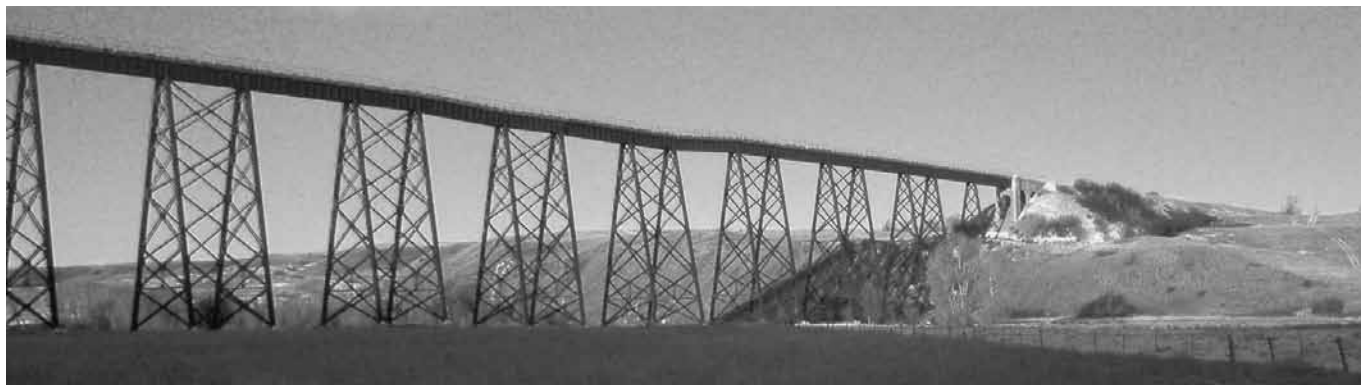
Figure 5. West half of Judith River trestle in 2011 after Judith River flooding damaged it (note misalignment of bridge spans).
