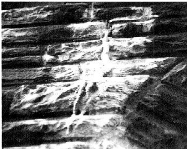
Figure 4. "Stalactite-like" formation, 24 inches in length, above arch in dam.
