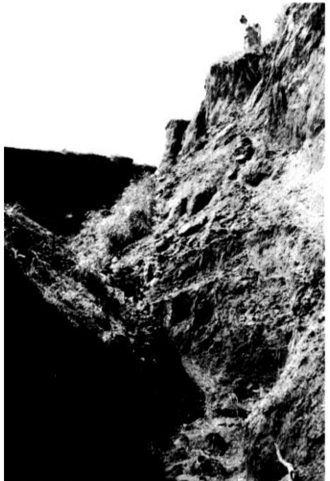
b. Looking up from the base of steep-sided gulley. Photographs by George F. Howe
