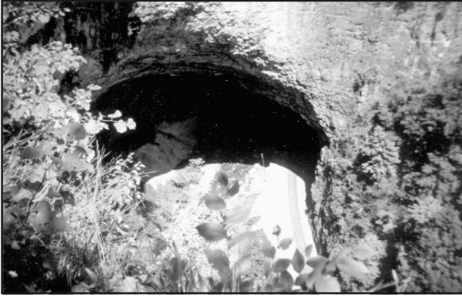
Figure 2. The south portal of Natural Tunnel. The Norfolk-Southern Railroad tracks are seen to the right. Stock Creek is to the left of the tracks. The trace of the Glenita fault is in the lower left of the tunnel. (Photograph taken in 1989)
