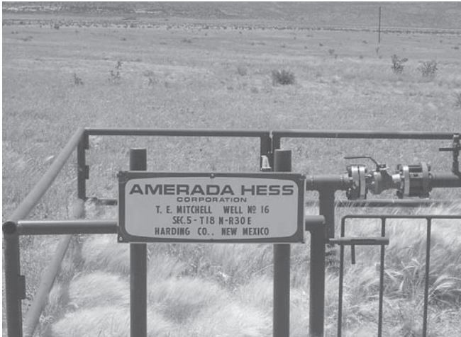
Figure 1. Bravo Dome Well Site (Mitchell #16) looking west. Sample point is the vertical pipe with valve on the far right.
