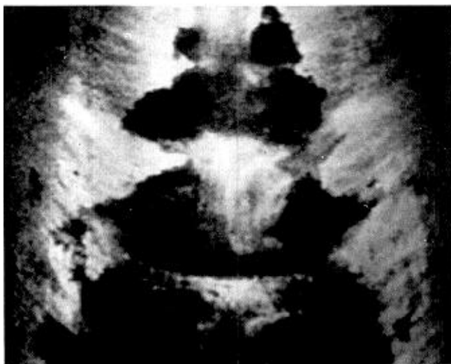
Figure 11. The first cavitation-induced holes in the left spillway were a series in which each one triggered the formation of the next. They were about 3 meters deep and 6 meters wide. (From Bureau of Reclamation video)
