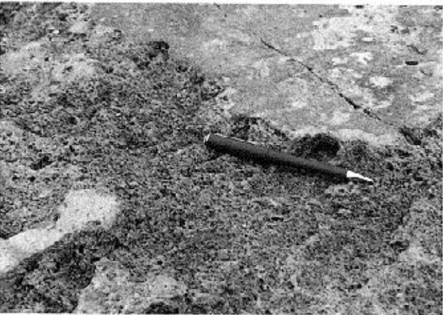
Figure 15. Pitted surface of limestone at Tuttle Creek Lake Spillway.
