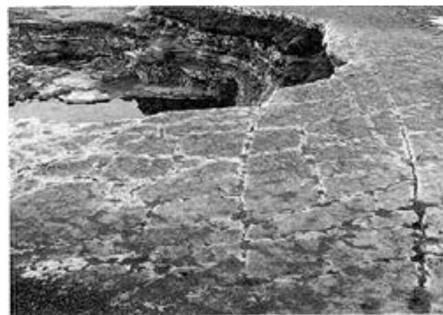
Figure 14. Cross joining of the limestone at Tuttle Creek Lake Spillway. Photographed area is that atop the ledge and to the right in Figure 9b.
