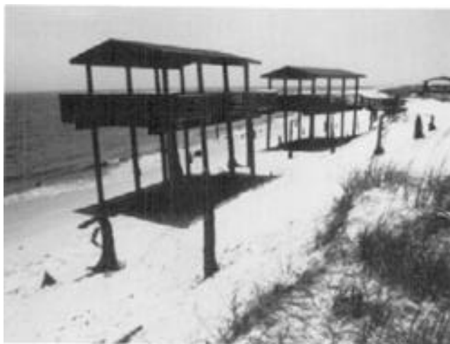
Figure 4. Low tide in June 1993. This photograph reveals tree stumps along the shoreline and the obvious loss of sand beneath the picnic areas. The picnic areas are approximately 12 to 14 feet above the beach.
