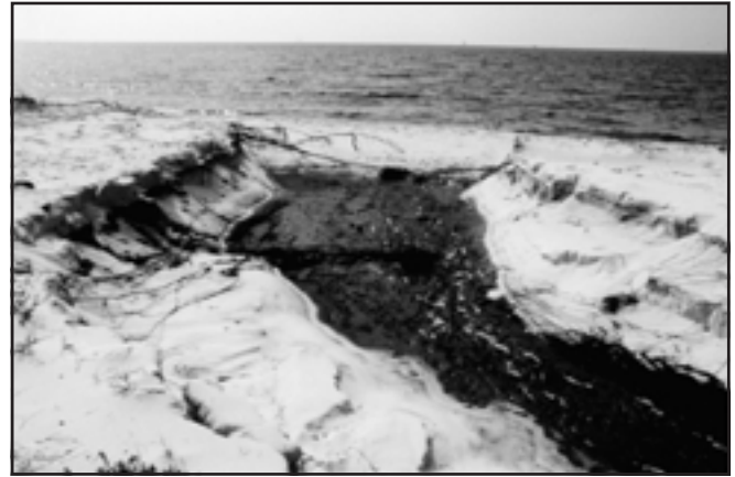
Figure 13. Another smaller washout channel area where the sand was discharged into the surf zone. Note the large pine tree root (approximately 1.5 inches in diameter) which still spans the channel. There is no evidence that sand accumulated in front of this area. Longshore currents in operation during the storm simply carried the discharged sands to the right and away from the front of this channel.
