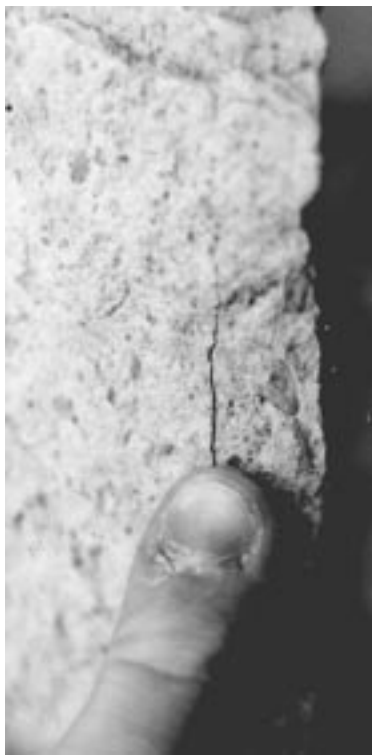
Figure 15. Oriented grains in a vertical sand-filled crack along the Hance Trail, South Rim. The crack edge is on the right.
