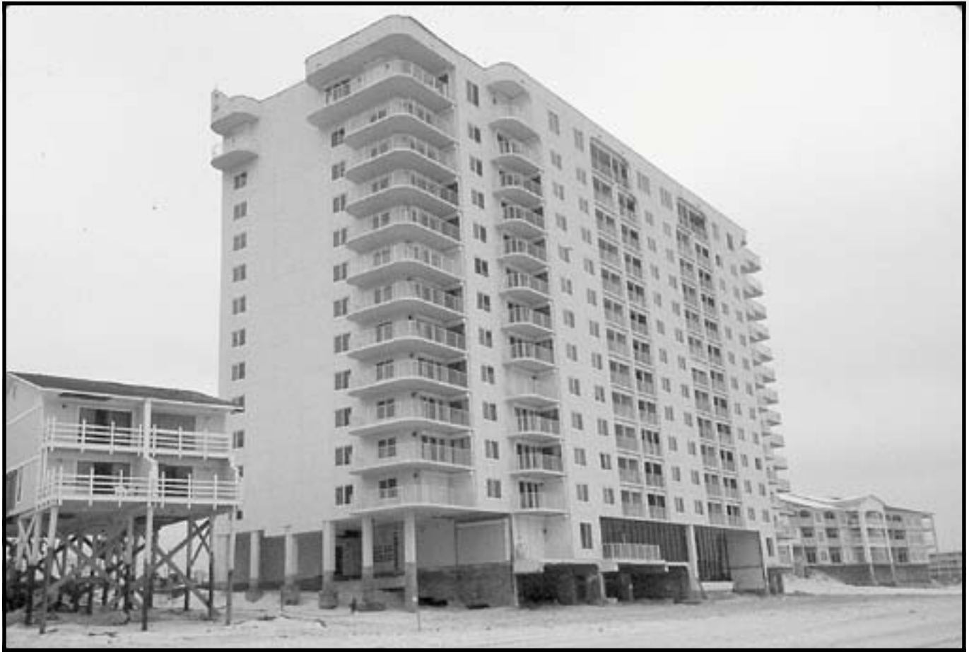
Figure 4. The footings of this large condominium are exposed due to the tremendous volume of sand removed from the beach by Hurricane Ivan. Approximately 10 to 15 feet of sand has been removed from beneath this building. Image taken on November 13, 2004.
