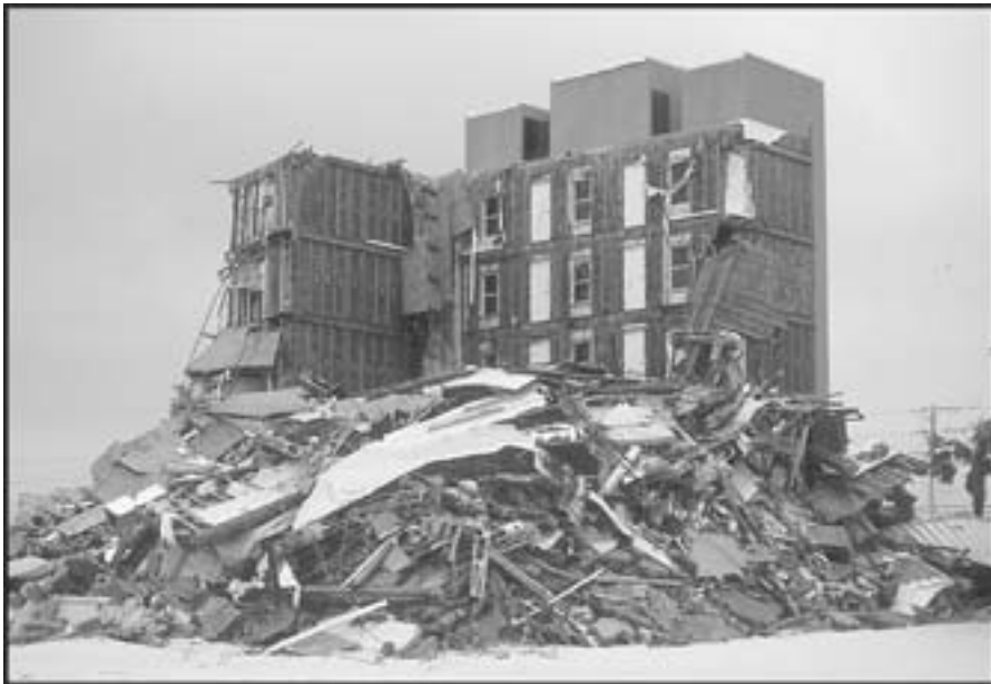
Figure 7. This image shows the damage to the large condominium shown on the left (indicated by black arrow) in Figures 5a and 5b. Apparently this structure was built on a concrete slab that was undermined during the course of the storm. Unable to retain its structural stability, a portion of the building collapsed. Note the exposed interior doors. Image taken November 13, 2004.
