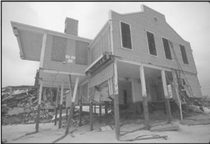
Figure 6. This image documents the loss of sand beneath this house constructed on piers. Note the white paint marking the former sand line. Approximately six to nine feet of sand has been removed from beneath this house. A portion of the beach-facing side (left) of the building has collapsed and was washed away during the storm. This is the small beach house on the right, shown in Figures 5a/5b, and indicated by a black arrow. Image taken on November 13, 2004.
