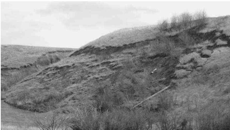
Figure 9. Small mass wasting events on the valley sides of the Ross Fork of the Judith River are relatively common.
