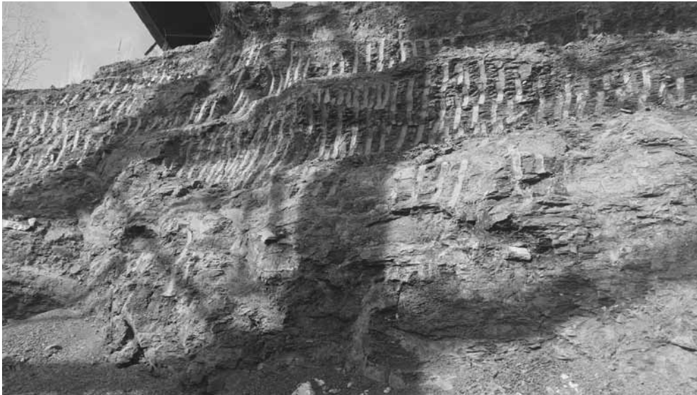
Figure 11 ( left ). The new bridge piers for the Ross Fork trestle are founded in freshly excavated bedrock of the Telegraph Creek Formation.
