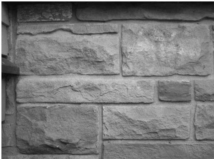
Figure 2. This 30-year-old reinforced stone foundation was built with upper Kootenai sandstone quarried 135 years ago, refaced, and reused. While the reinforced concrete piers and grade beams it sits on have an unconfined compressive strength of 5,000 psi (34 MPa), the sandstone averages 11,000 psi (75 MPa). The primary stone is a medium-bedded arkosic sandstone (immature, fine-grained to medium-grained subarkose) with minor iron cement; some of the stone is argillaceous (sublitharenite) but it still exhibits a strength of at least 7,000 psi (48 MPa).
