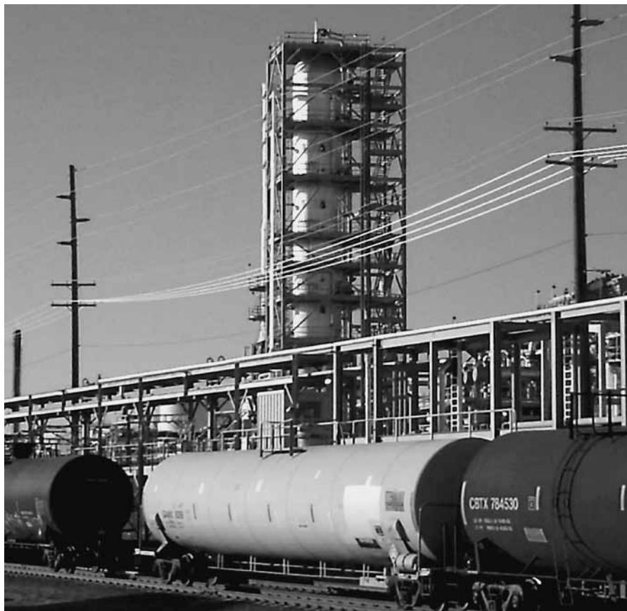
Figure 1. The foundation for the 6,000-ton catalytic cracker in the center of this picture is founded 13.7 m (45 ft.) into upper Kootenai Formation sedimentary bedrock to prevent even a few millimeters of differential settlement. The bedrock consists predominantly of claystone with sandstone interbeds (fine-grained, argillaceous sandstones).
