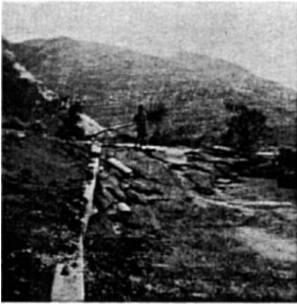
Figure 8. Overall view of twisting and faulting in blacktop of Blue Star Trailer Court, San Fernando, California. The fracturing, slanting, and toppled nature of the blacktop would in itself be evidence of overthrusting.
