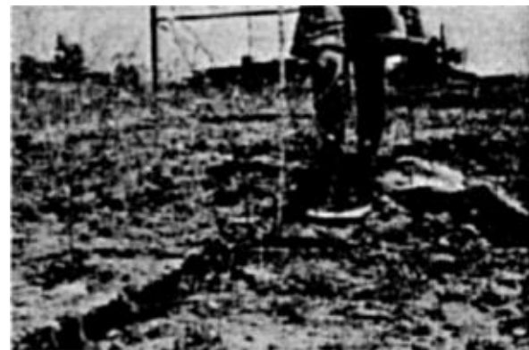
Figure 3. Interstate 210 fault line in clay road bank. North and east of the highway the fault line is visible in the earth fill. There is no evidence of overthrusting in this soft material although the one side of the fissure is now about six inches higher than the other.
