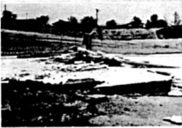
Figure 1. Interstate 210 fault line in concrete: overall view. As the concrete was broken, whole slabs were shoved across other slabs during the earthquake. Barbara Howe is seen in this and other photographs.
