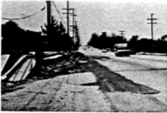
Figure 4. Foothill Boulevard fault escarpment. Here the actual fault line can no longer be seen because of road repair. It is obvious, however, that the sidewalk was elevated several feet in relation to the road bed. This view is toward the southwest, along the fault.
