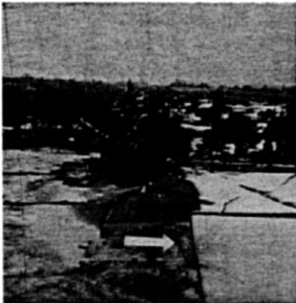
Figure 9. A blacktop, concrete overthrust. Philip Howe is standing on a blacktop slab which was moved some three feet laterally southwestward (direction of superimposed arrow) during the San Fernando earthquake. This is an example of a soft material (asphalt) moving over a harder material (concrete).
